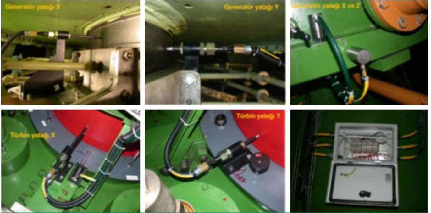
Figure 13. Placement of the sensors used in generator and turbine bearings
